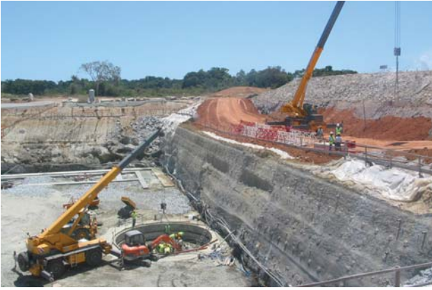
Excavation of the large Russian-style flame duct for the new Soyuz Launch Complex (ELS) at Europe's Spaceport in Kourou (Fr. Guiana) in March (Photo: ESA/CNES - Photo Optique Video CSG)
